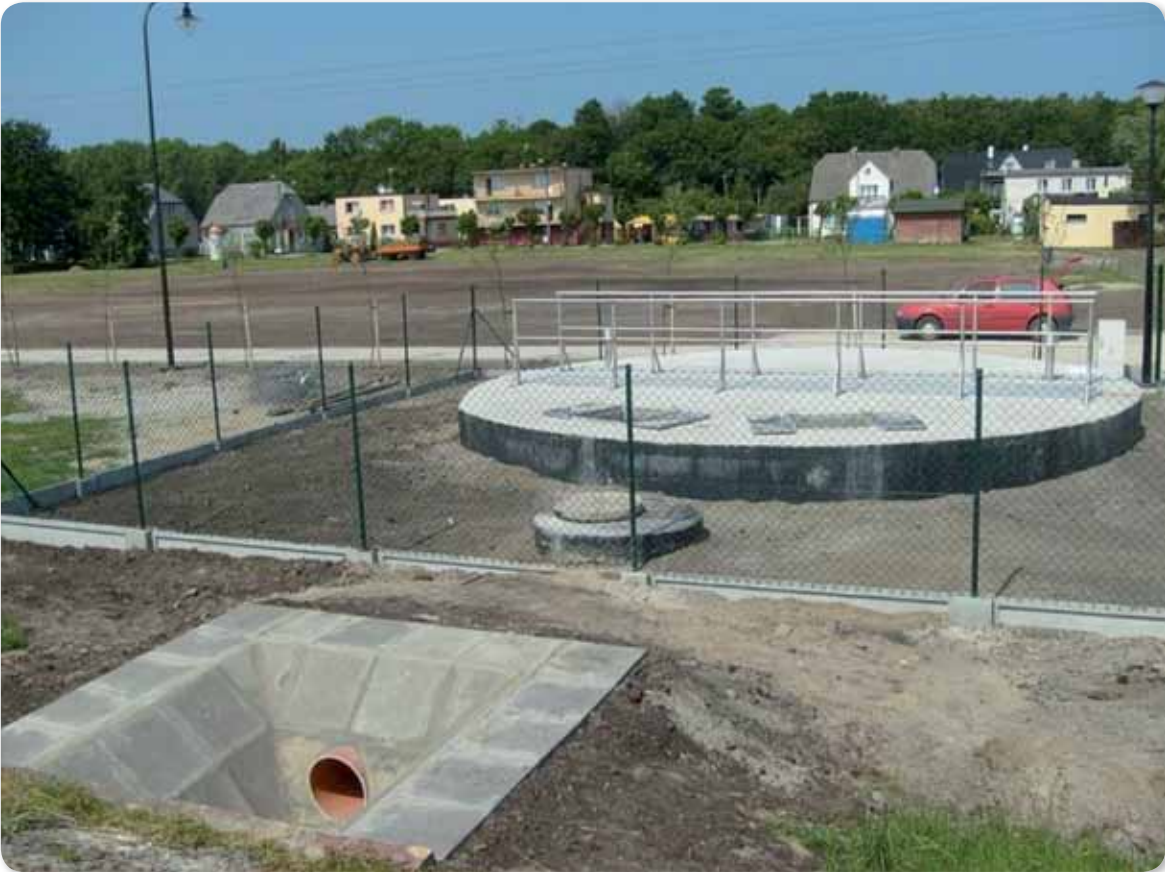
Chalupy pumping station EPS
