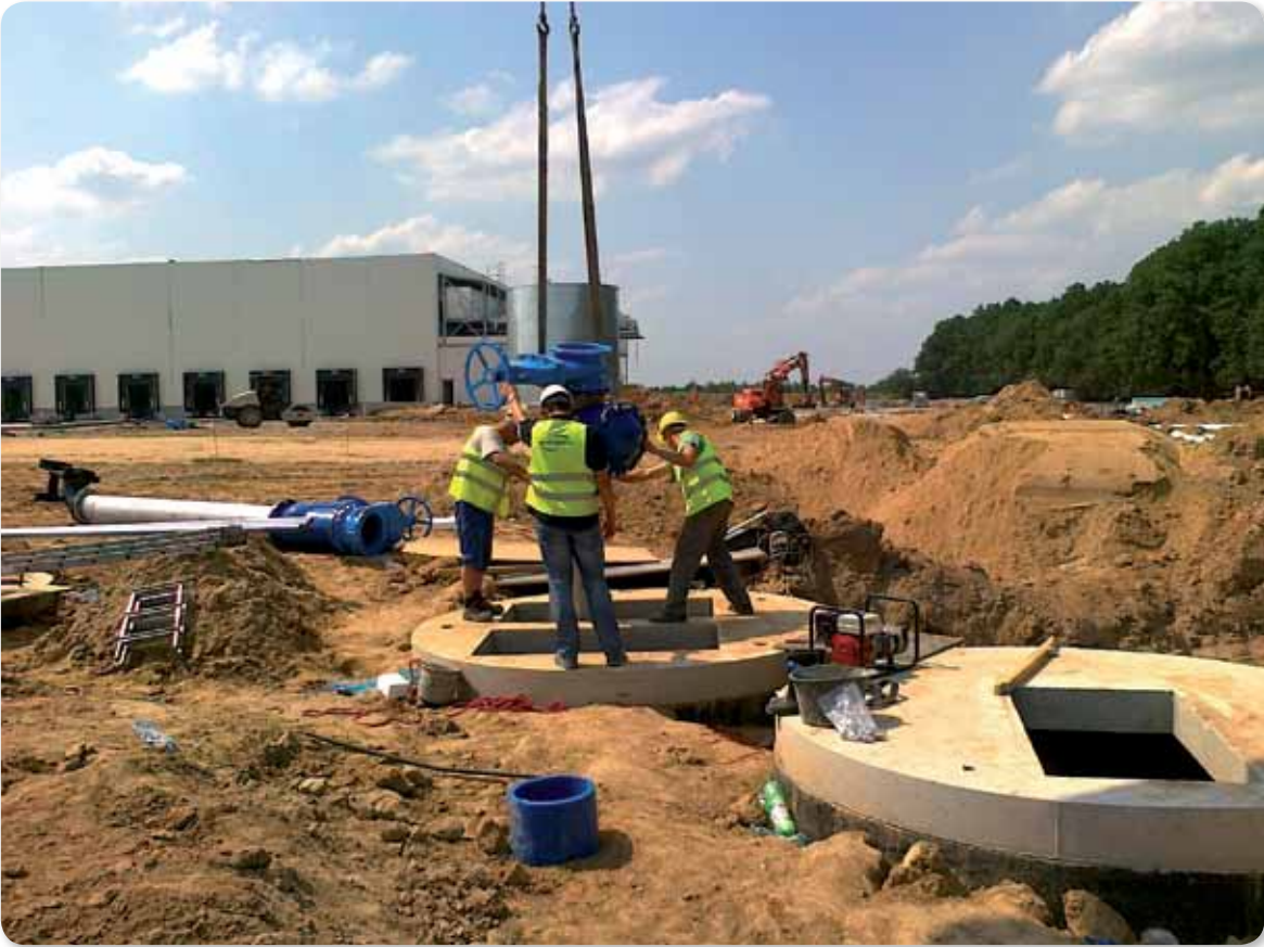
Biedronka's Logistic Centre, Sieradz pumping stations EPS, EU chambers
