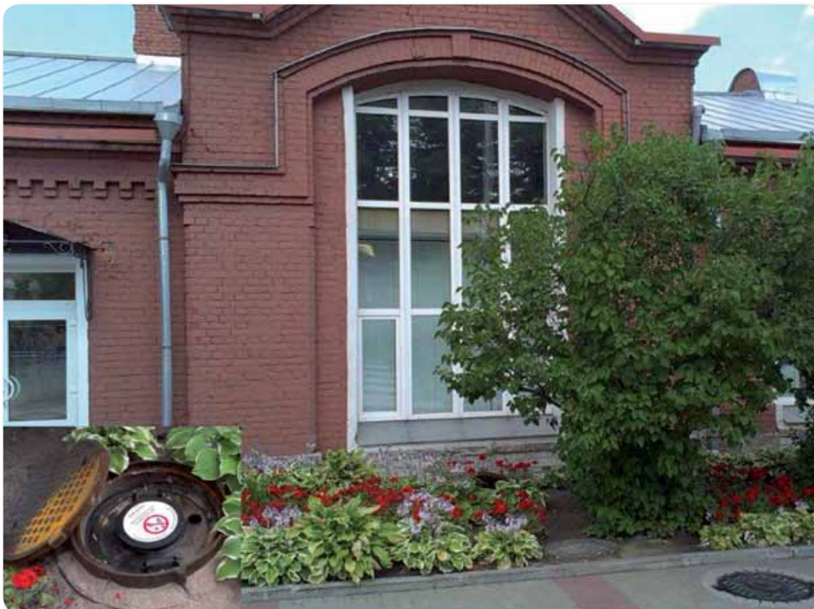
Water and sewerage company, St. Petersburg Anti-odour filter EMF
