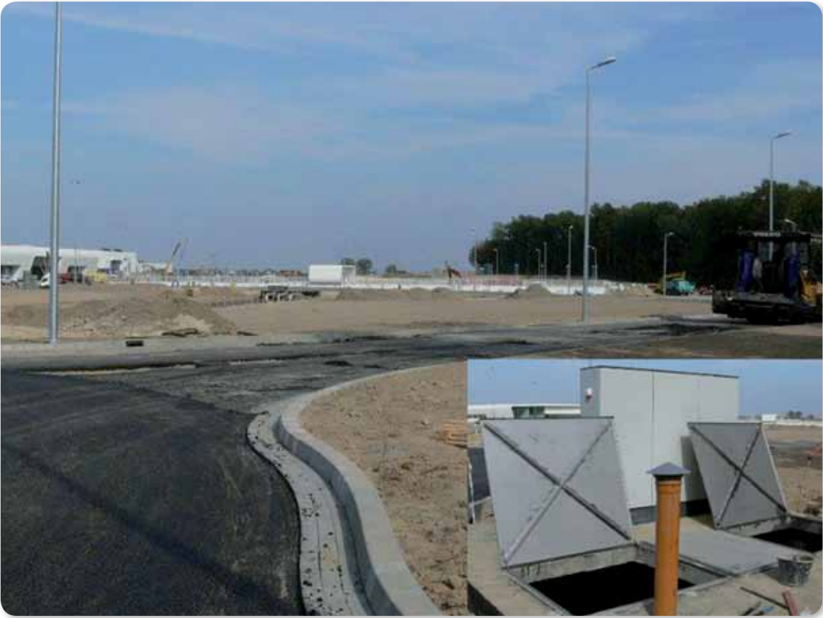
Swidnik Airport pumping stations EPS, separators, settling tanks
