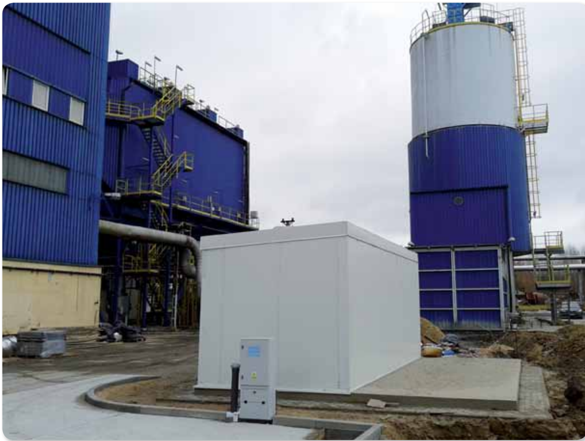
Zgierz Thermal Power Station pumping stations, flow regulators, EU chambers
