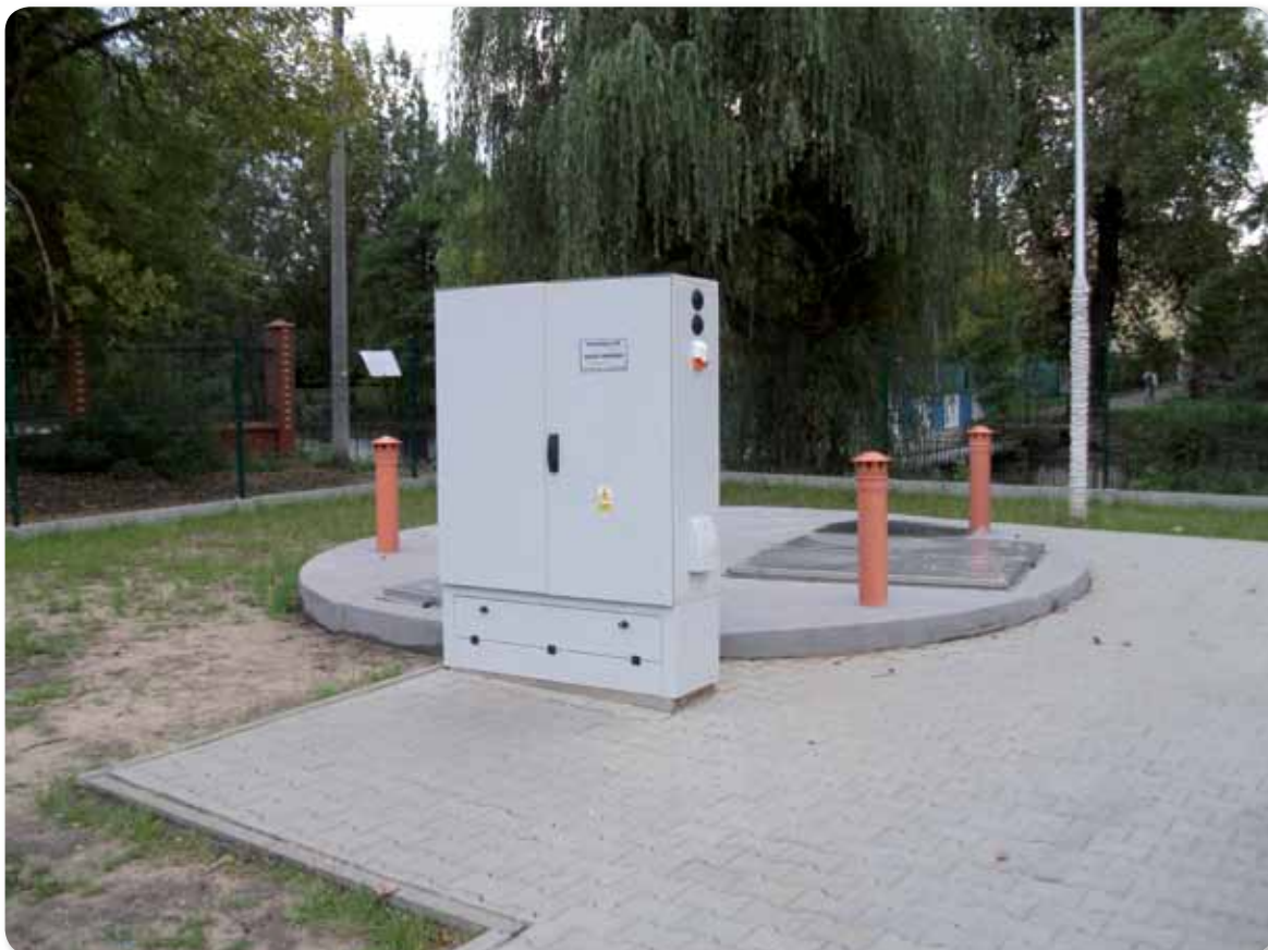
Katowice Sewerage System dry well pumping station with solids separation systems ETS
